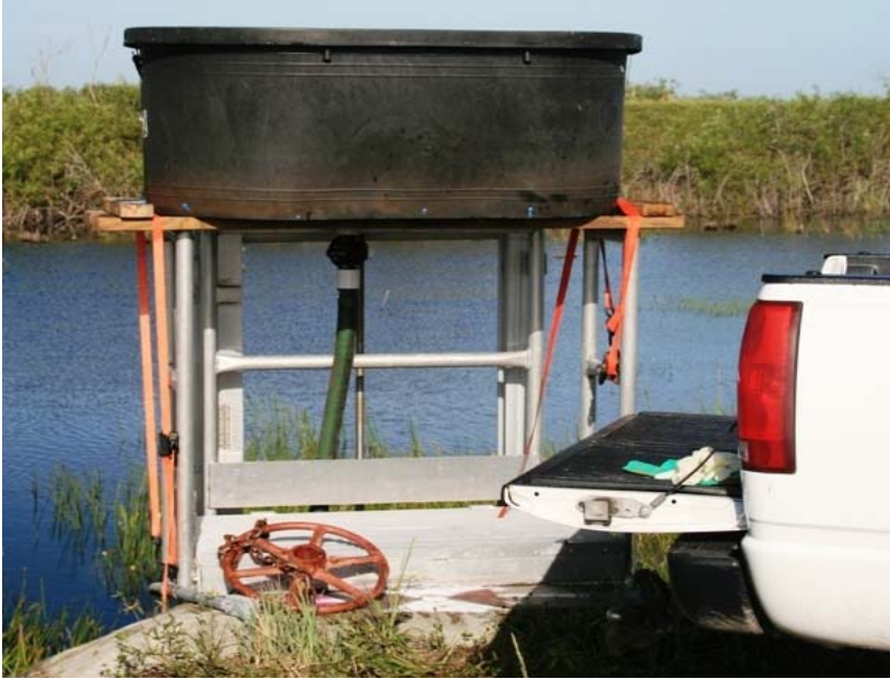
Figure. 6.2.5.2. Dye injector - note valve below mixing tank that allows for constant flow.
